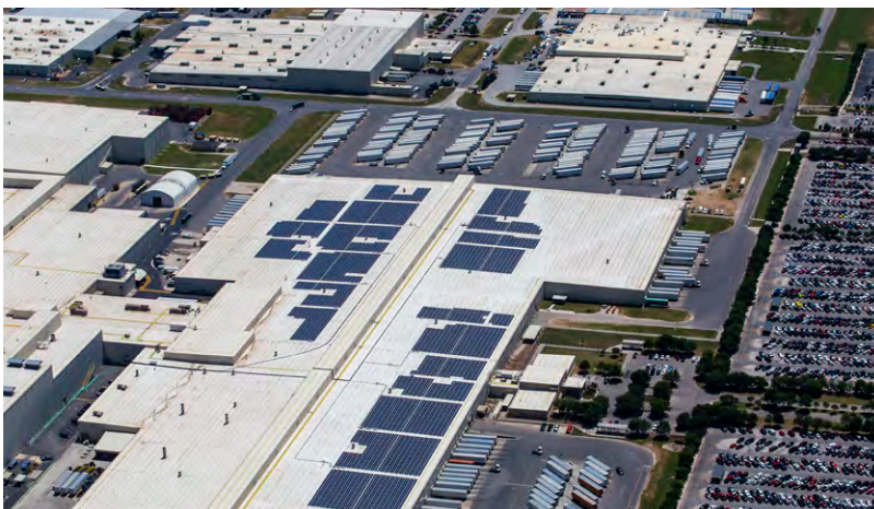
A 3.1 megawatt solar array was also installed on the roof of the assembly plant building. These panels are expected to generate around 3 percent of the plant’s annual demand.
